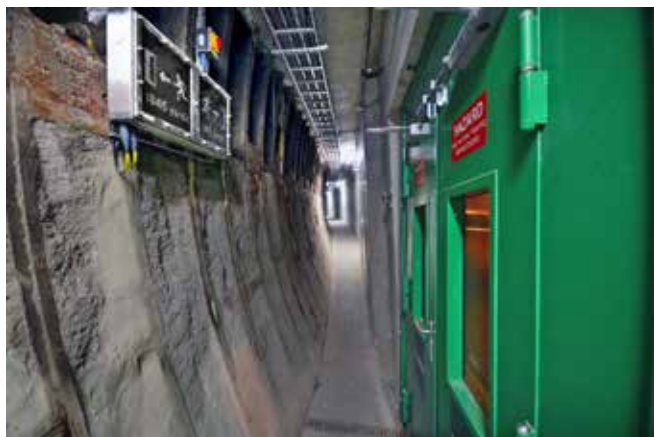
Inside the newly-built narrow escape gallery in the northbound Tyne Tunnel as traffic streaks by beyond the green emergency doors. The escape distance sign is in yards as tunnel speeds are in miles per hour
